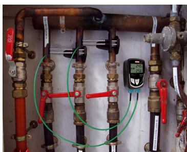
To prevent legionnaire's disease : check of hot water sanitary network
